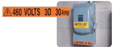
Electrical Panel ID
